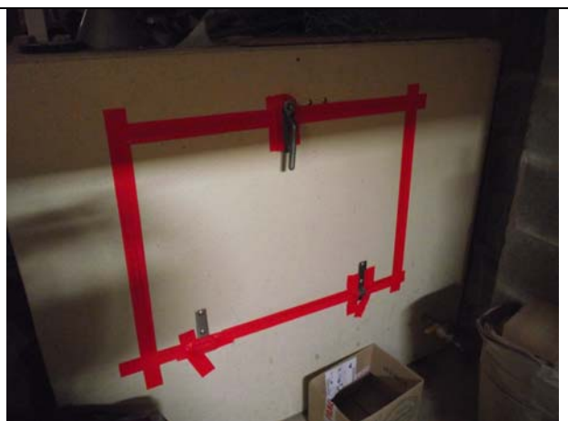
Hatch to composting chamber temporarily sealed with tape awaiting the fitting of effective & robust draughtseals
