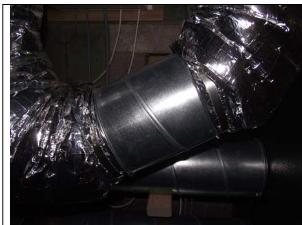
Supply and return ducts disconnected from warm side of heat exchanger and temporarily joined for the duration of testing
